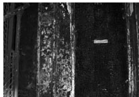
Fire damage at Evelyn Court
