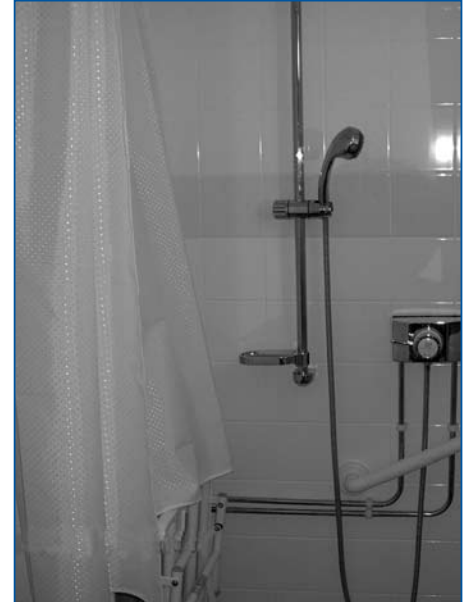
Level access shower fitted in one of the tenants flat.
